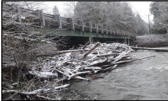
South Skagit Highway at Finney Creek
