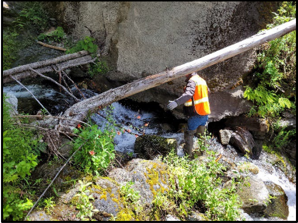
Scoured channel bank undermining retaining wall along east bank.
