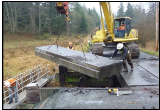
Campbell Lake Outlet slab girders put back in place after receiving new timber cap in 2013.
