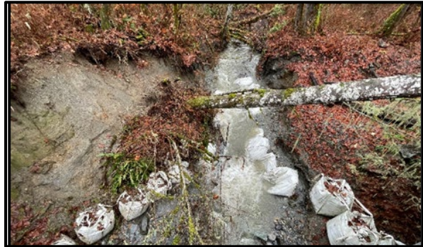
Super-sacks filled with river rock are placed to armor bank and slow down channel migration. Photo taken from bridge looking upstream.
